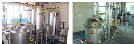
Figure 2: Pretreatment plants with 100 L-Reactor (left) and 425 L-Reactor (right).
